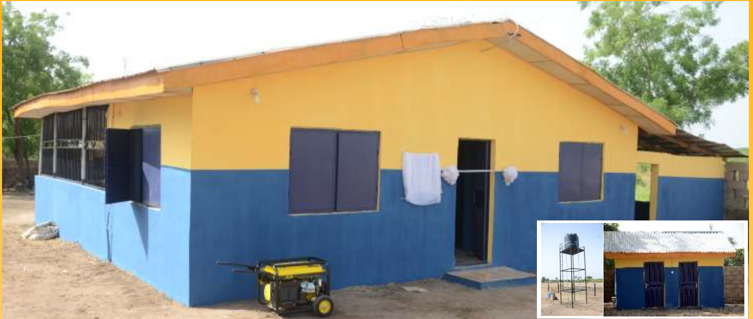
The rehabilitated cassava processing cottage Industry. Insert are the water and sanitary facilities provided to improve hygiene at the industry and serve the community.
